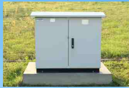
Electrical feeder pillar
